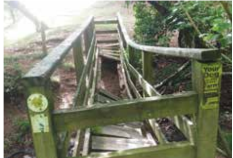
Footbridge in south-west Herefordshire, closed since August 2020 by a TTRO because the council has failed to mend it. Photo: David Howerski.
